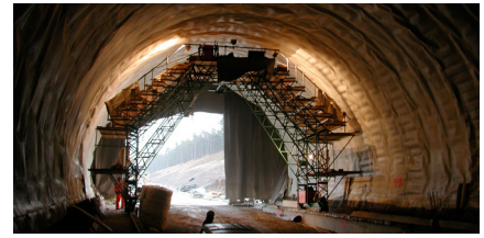
[Tunnel Application, Germany]
