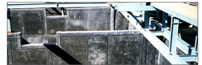
[GSE Liner in wastewater treatment aerobic digester]
