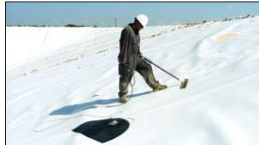
GSE Conductive spark testing can be performed with hand-held equipment.
