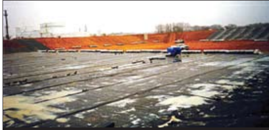
GSE GundSeal deployed as a composite liner in a food processing sludge lagoon.
